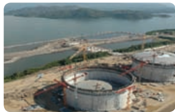
▼ The Construction Site of LNG Terminal in Manzanillo, Mexico ▼▼ The Dedication Ceremony of LNG Terminal in Manzanillo, Mexico with the President of Mexico
